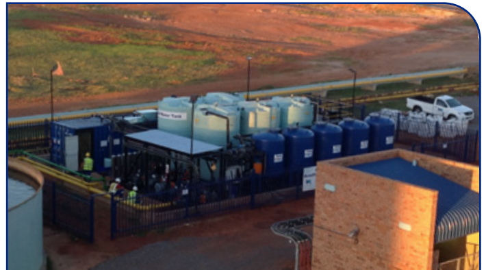
2.5 ML/DAY EXCESS UNDERGROUND MINING WATER TO POTABLE DRINKING WATER PLANT
