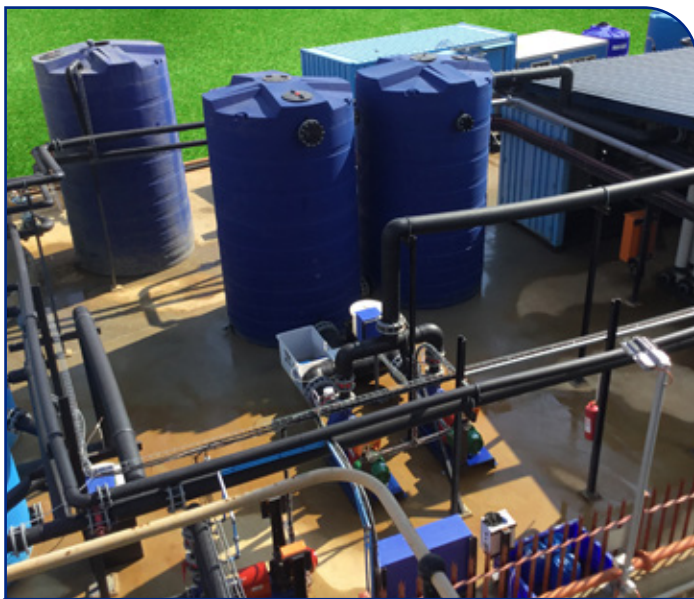
4.5 ML/DAY EXCESS UNDERGROUND MINING WATER TO POTABLE DRINKING WATER PLANT
