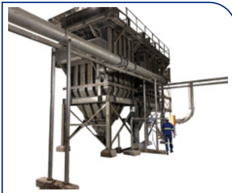
HIGH RATE CLARIFIER
